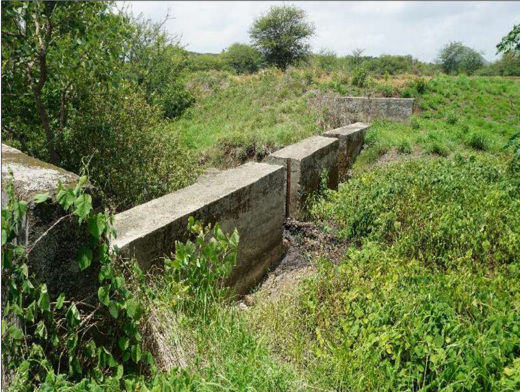
Photo 36: No gates to gated checkdam therefore no water
