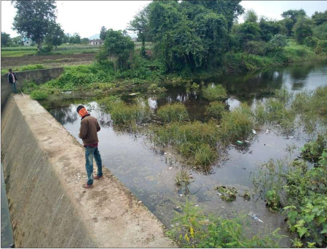
Photo 35: Checkdam silted by reducing the storage capacity
