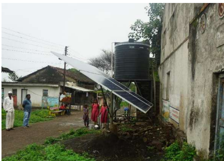
Photo 31: Solar-powered unit for drinking water supply in Khatawad village
